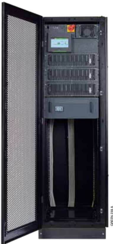
Example of integration (3x25 kW). Only 15 U of rack space occupied: space-saving design leaving free space for other rack-mounted devices. One empty slot in the MODULYS RM GP sub-rack remains available for power upgrade or redundancy.
